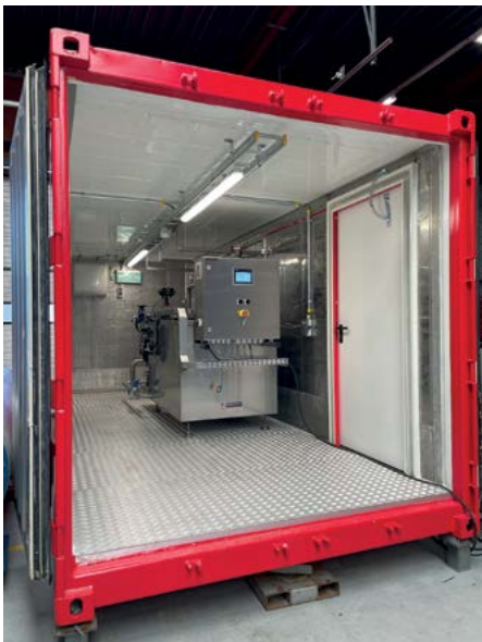
The equipment used for the tank cleaning facility in Gothenburg
