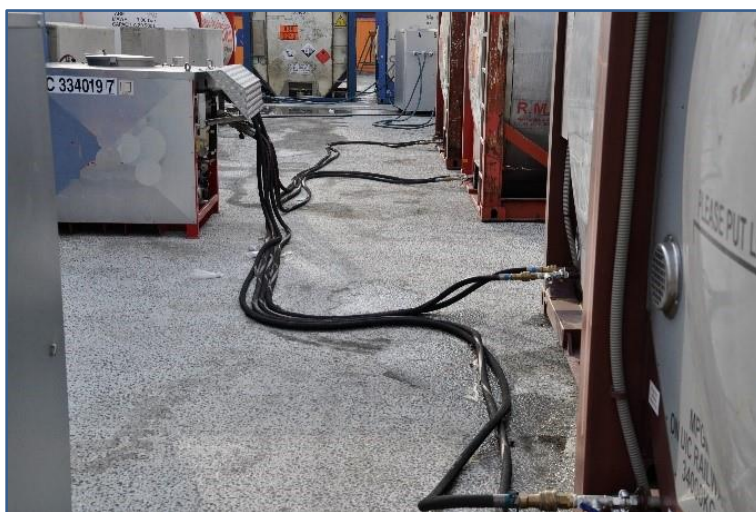
Figure 14 - Containers connected to a heating unit
